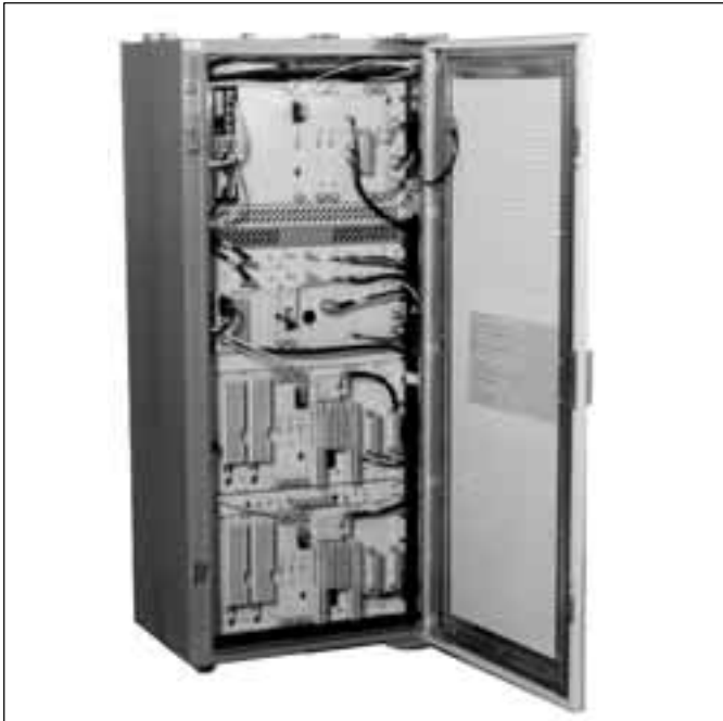
Base station of cellular network
